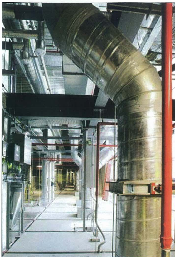
Walkable ceilings minimize traffic in cleanrooms.
