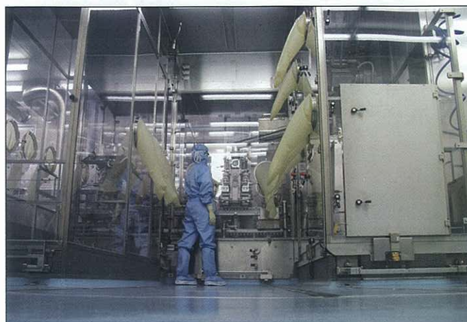
Core of the aseptic area.
