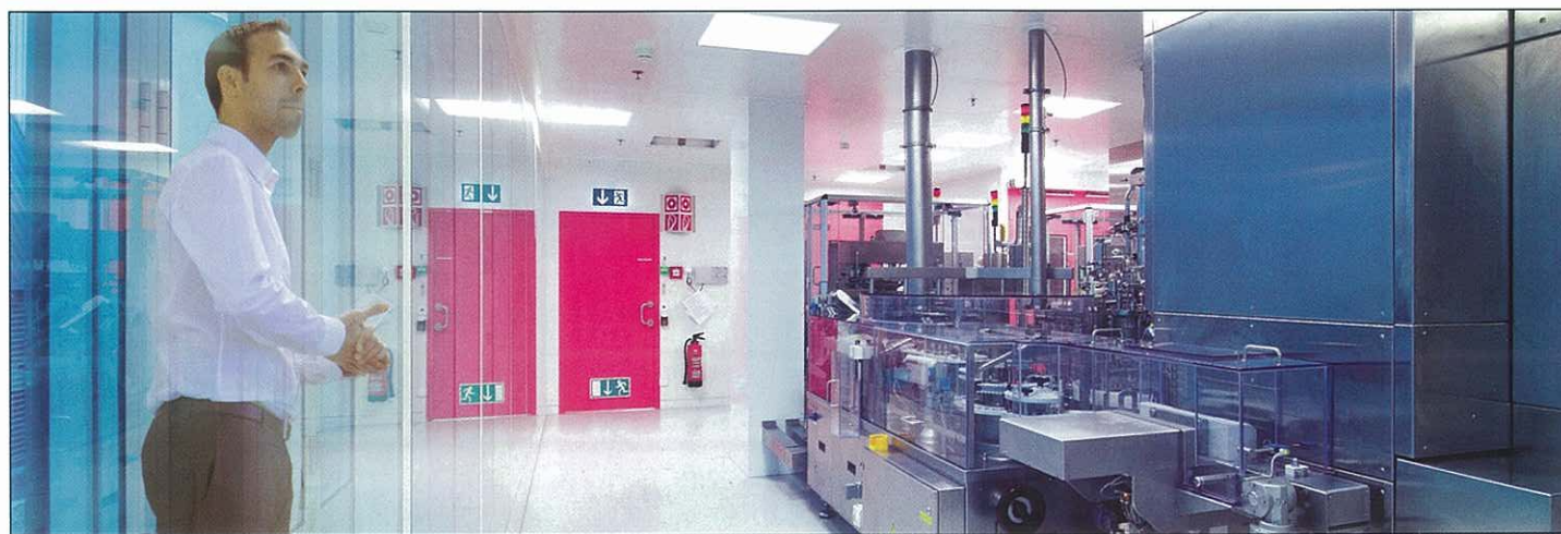
View from the visitor corridor of the washer and depyrogenation tunnel located in the C-grade area.
