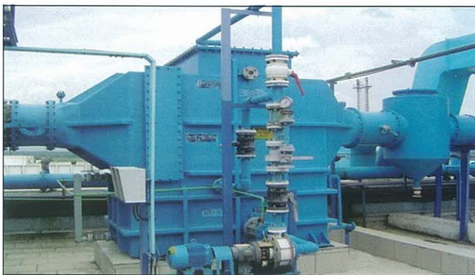
Horizontal scrubbing system.
