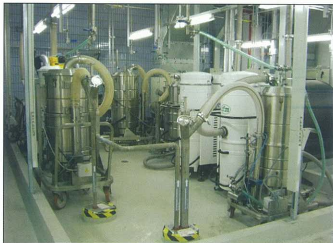
Wet dedusting systems.
