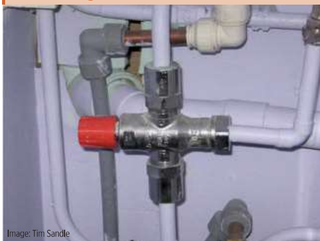
Figure 3: Poorly designed water distribution pipe with a dead leg
